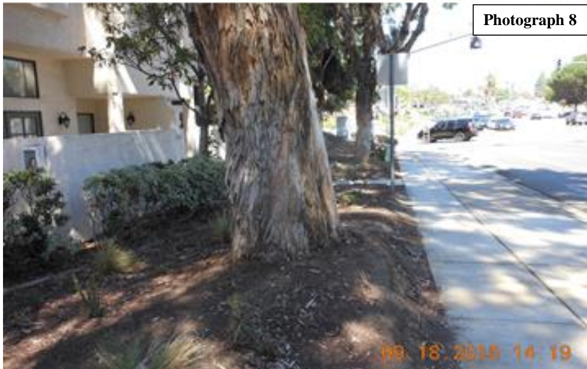
Photographs 7 (top) and 8 (above) show a section of subject East H Street eucalyptus trees and their proximity to the adjacent sidewalk. The trees are located less than three feet from the adjacent sidewalk.
