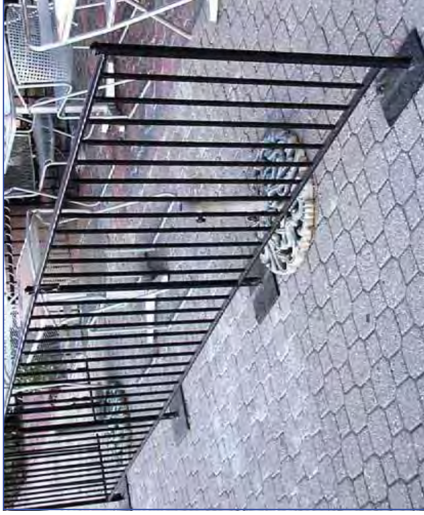
Figure 2: Acceptable use of a sectional fence. Note appropriate base and connection to the fence.
