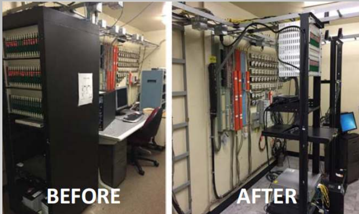
Traffic Signal Communications Center (TSCC) Upgrade
