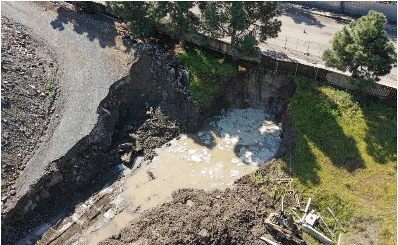
Figure 1 – Drone Aerial Photo of 855 Energy Way Sinkhole
