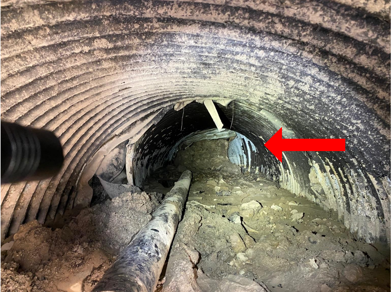
Figure 5 - Additional CMP Failure Discovered Downstream of the Excavation Pit
