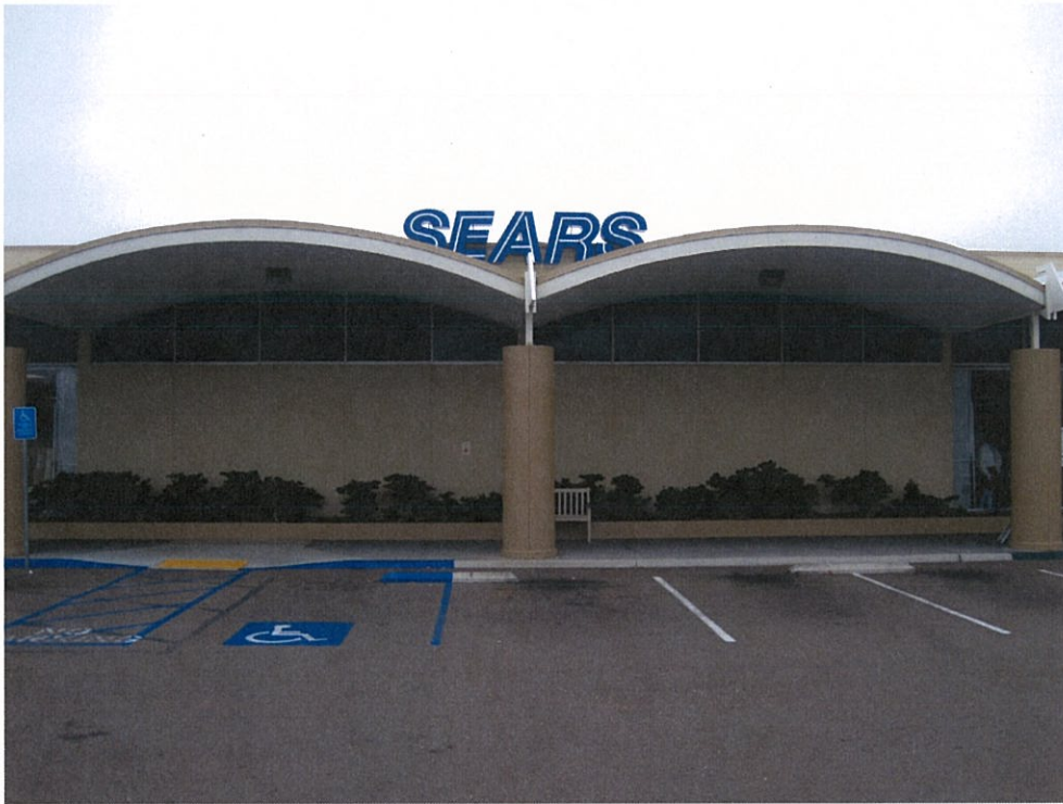
Figure 2-10: Detail of the barrel roof canopy, retrofitted posts, and enclosed original display windows at the south entry.
