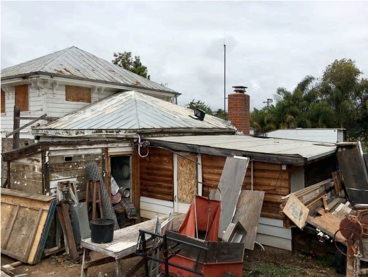
Photo 6: View northwesterly of the east wing, southeast corner, with the shed roof addition in the foreground.
